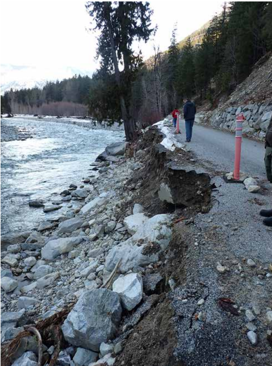
2025 flood damage to the Stehekin Road. —PAUL BAKKE PHOTO
