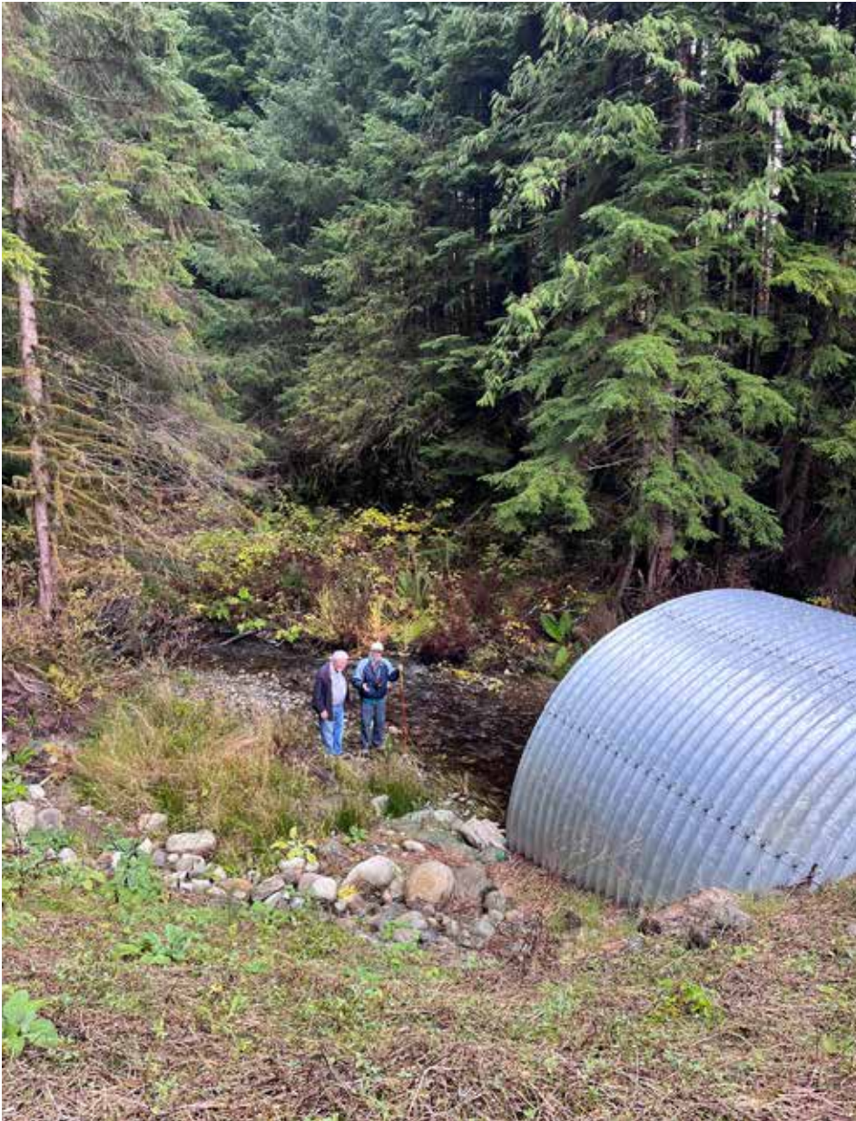
A huge new culvert that replaced a small one as part of stewardship work. Large culverts like this allow streams to carry aquatic organisms including fish that were previously blocked by small culverts. —PHIL FENNER PHOTO
